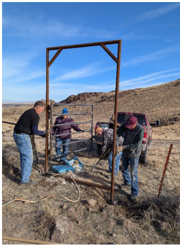
Boise Back Country Horsemen - Installing ride-through gates in the Wilson Creek Travel Management Area.
