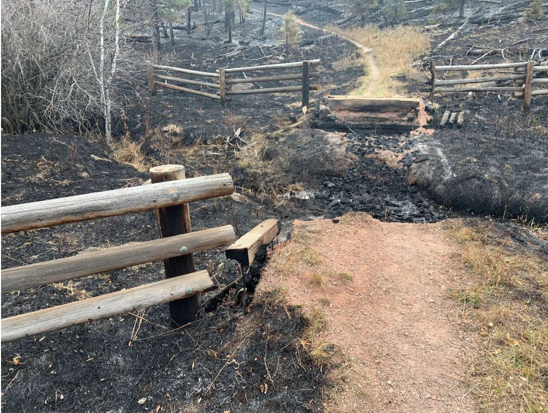
Figure 16. Palmer Creek bridge immediately after wildfire in 2022.
